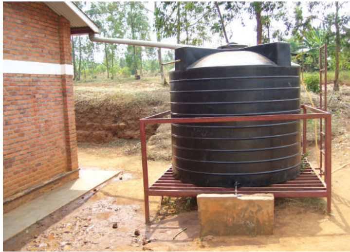
Fig 9.6: A water tank
