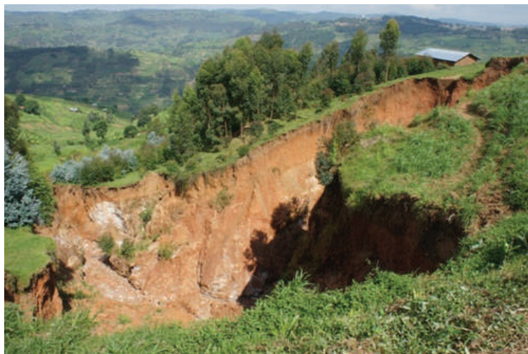
Fig. 5.8: Large gully at the edge of the Gihembe Refugee Camp caused by soil erosion
